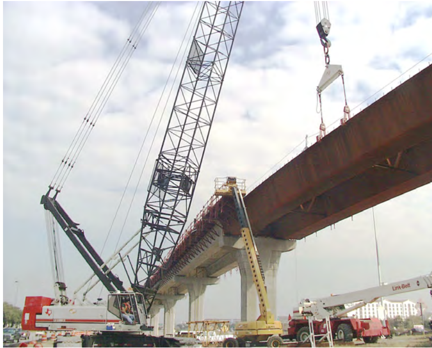
Figure 3.4 Loading Crane & Top-Flange Attachment
