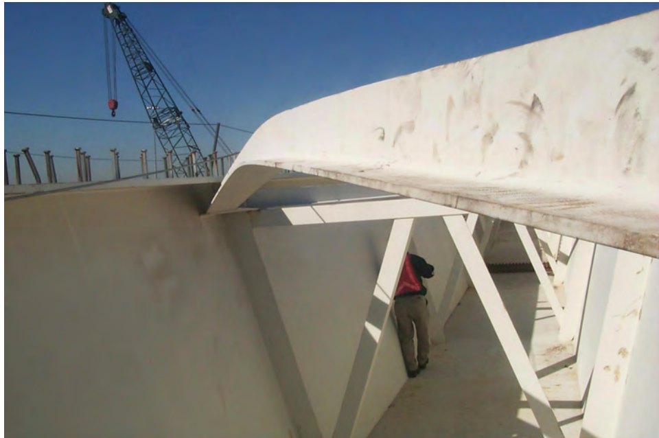
Figure 1.4 Failure of Top-Lateral Brace During Bridge Erection (T. Helwig, U. of Houston)
