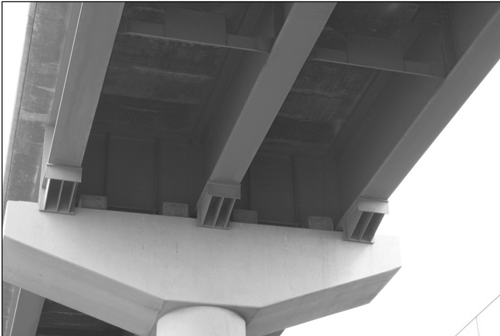
Figure A.9 Site photograph of fixed bearing condition at bent 9 of curved bridge
