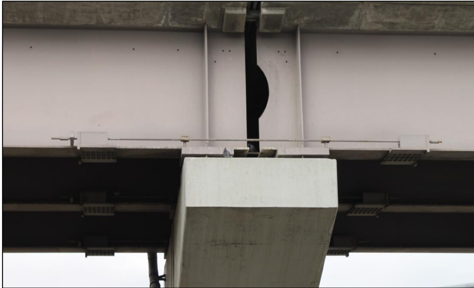
Figure 2.5 Restrainer rods at expansion joints of curved bridge
