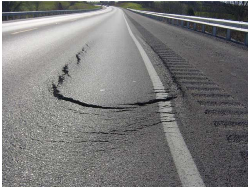
Figure 2.3: Slippage cracking after overlay construction (Buchanan and Woods 2004).
