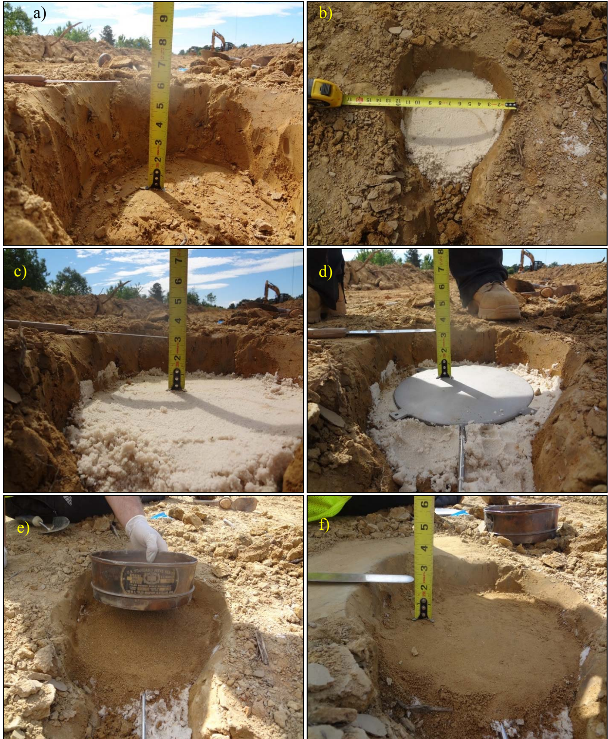
Figure 3-7. a) Depth of the EPC below the stabilized layer; b) 10”~11” hole; c, d) 3” hand-compacted silica sand; and e, f) 1” soil (fraction that passed sieve No. 10).
