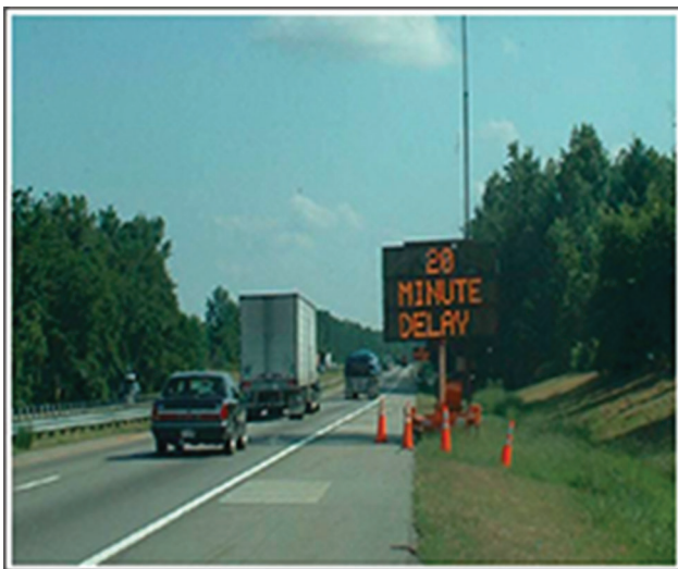
Figure 3.19 Roadside message sign providing delay information (Bushman & Berthelot, 2005).
