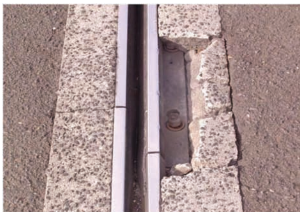
A.1.1. Significant Spall
