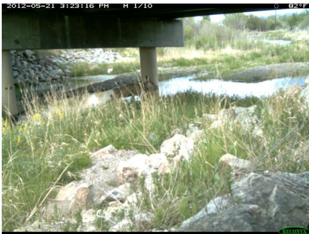
Appendix K, Figure 20: Underpass south of Madison River Bridge at Ennis, US 287 - camera image (project photo).
