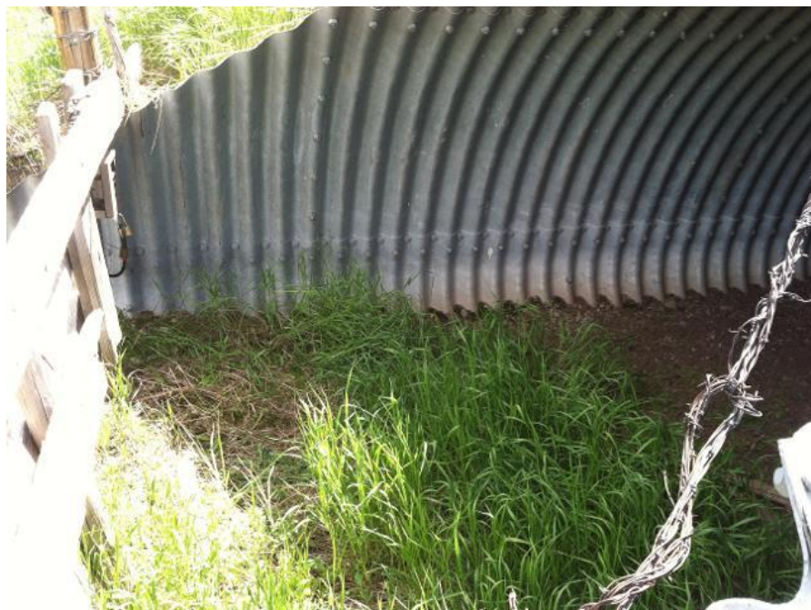
Appendix K, Figure 3: Stock culvert at RP 5.2, MT 87 -- Camera location (Photo courtesy of Lance Craighead, CHI)
