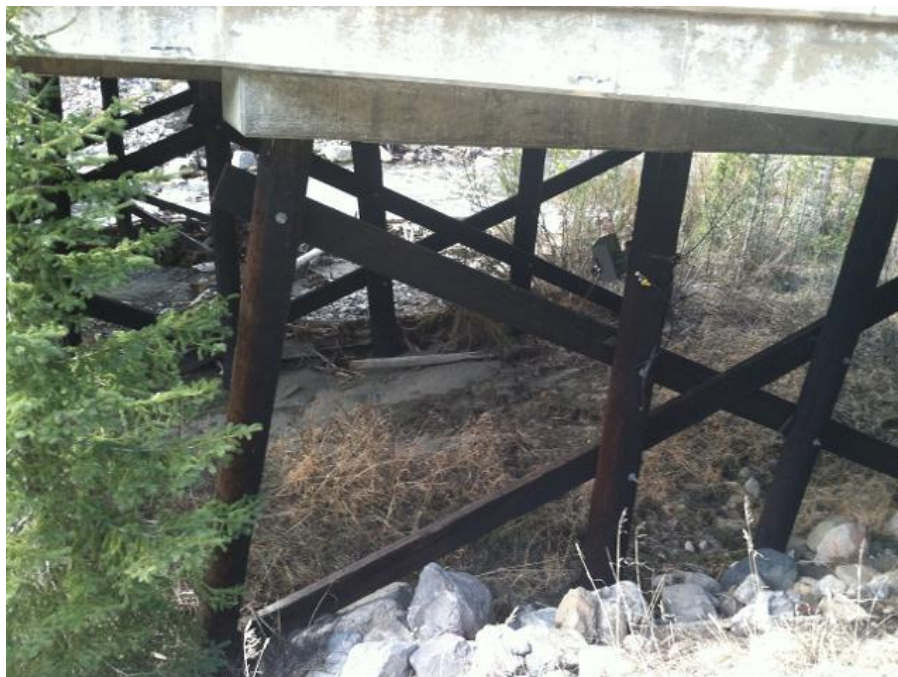
Appendix K, Figure 9: Beaver Creek Bridge (east) - camera location (photo courtesy of Lance Craighead, CrI).
