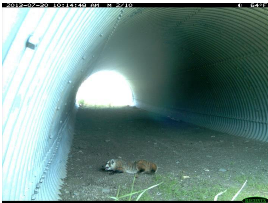
Appendix K, Figure 4: Stock culvert at RP 5.2, MT 87 -- Camera image (project photo)
