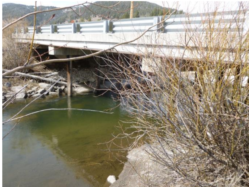
Appendix K, Figure 13: Grayling Creek Bridge, US 287 - camera location. Note: the camera is not visible in this photo, but is located at the southwest corner under the bridge, which correlates to the upper right quadrant of this photo (Photo courtesy of Lance Craighead, CrI).
