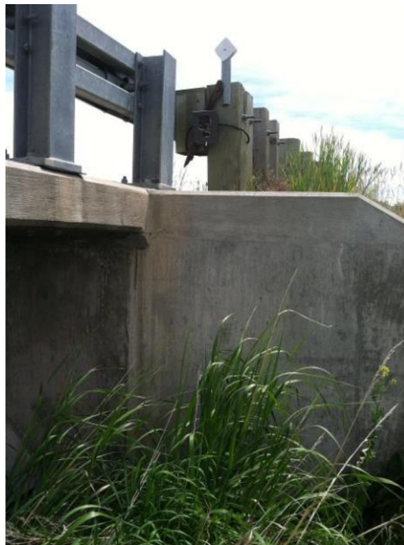
Appendix K, Figure 17: Madison River Bridge at Ennis, US 287 - camera location (photo courtesy of Lance Craighead, CrI).
