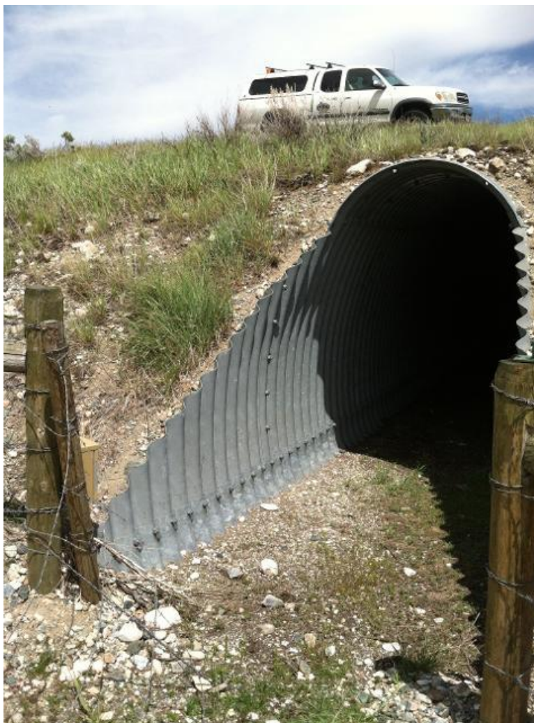
Appendix K, Figure 1: Stock culvert at RP 3.5, MT 87 -- Camera location (Photo courtesy of Lance Craighead, ChI)
