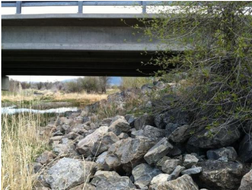
Appendix K, Figure 19: Underpass south of Madison River Bridge at Ennis, US 287 - camera location (photo courtesy of Lance Craighead, CrI).
