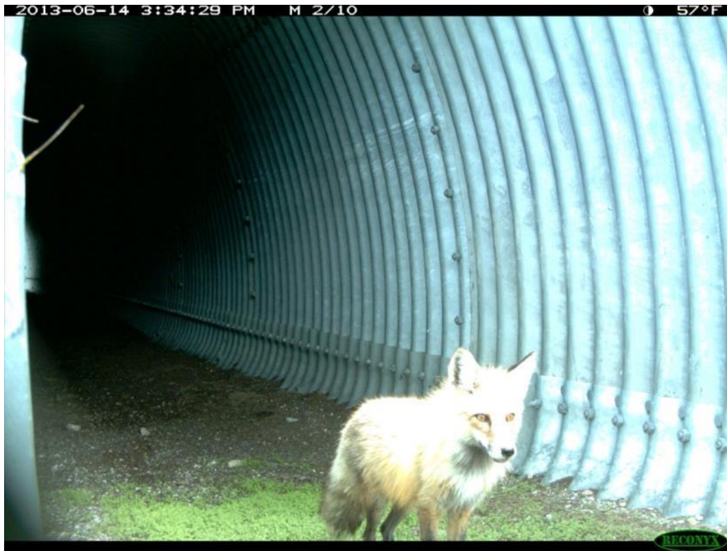
Appendix K, Figure 2: Stock culvert at RP 3.5, MT 87 -- Camera image (project photo)
