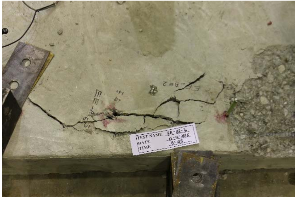
Figure B.60 Specimen details after testing for EE-AE-3
