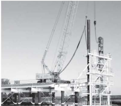
Figure 1. Photo of a temporary pile being driven by a hydraulic impact hammer during construction of a highway bridge in Queensland, Australia (from Erbe 2009).
