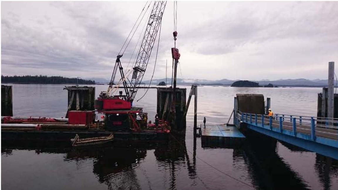
Vibratory extraction at the east side of the Kake Ferry terminal (JASCO Applied Sciences, September 2015).
