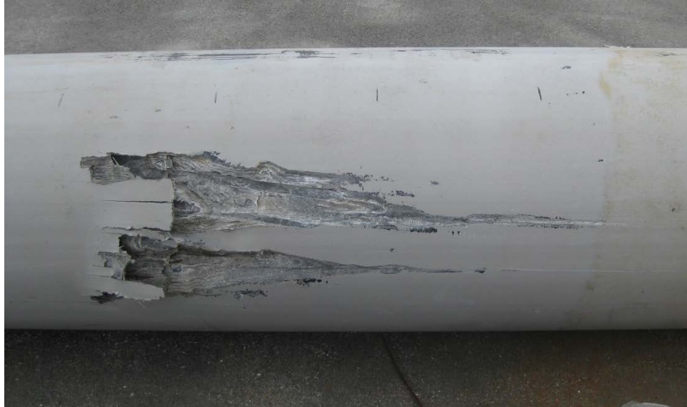
Figure 5.9 Damage to Pile D from Pile Extraction
