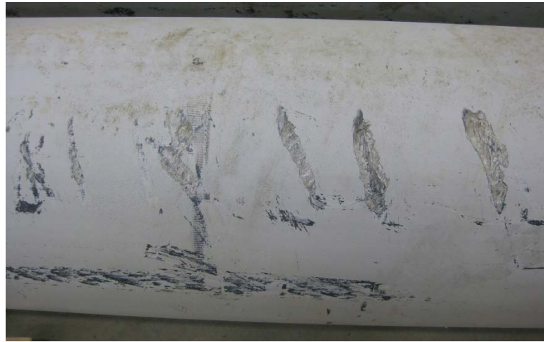
Figure 4.9 Typical Damage Due to Pile Driving/Extraction
