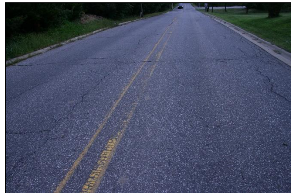
Transverse and Longitudinal Cracking
