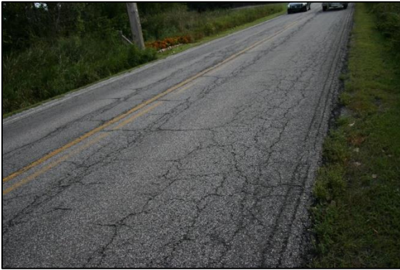
Fatigue cracking along wheel path
