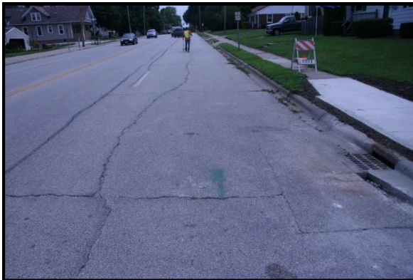
Transverse and Longitudinal Cracking
