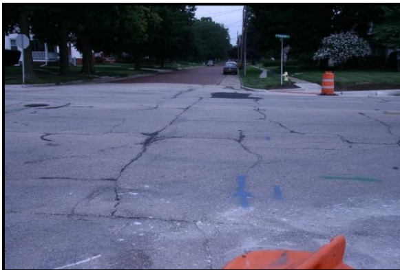
Block Cracking at Intersections
