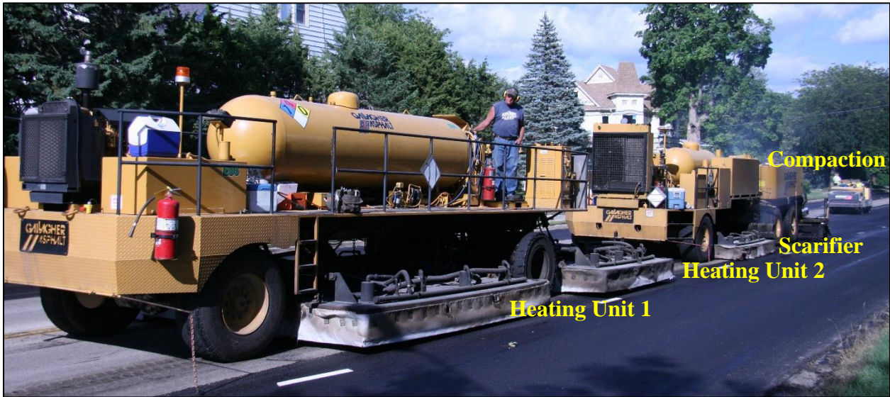
Figure 3-3 HIR construction train showing two heating unit and scarifier followed by compactor
