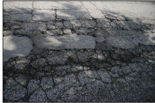
Severe Fatigue Cracking
