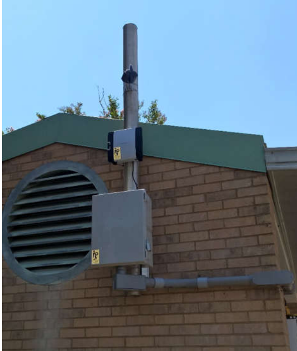
Figure 12. Installed site controller
