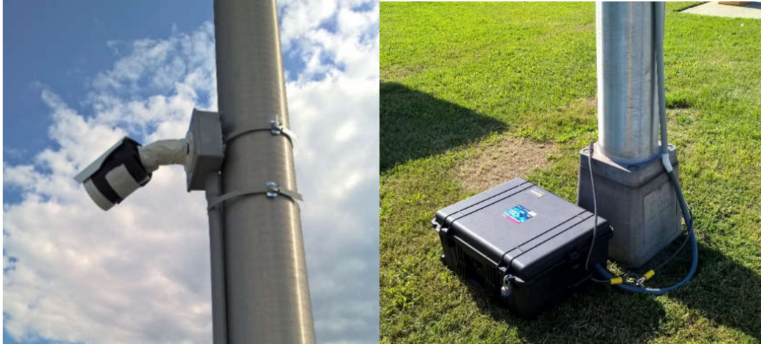
Figure 22. Installed camera, PVC conduit, and Pelican case
