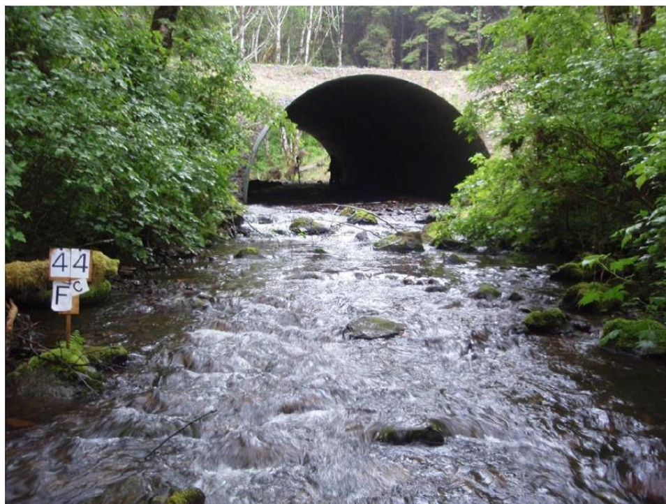
Figure 3.1: Culvert for AOP, which mimics the natural bedstream (from Barnard et al. 2013).
