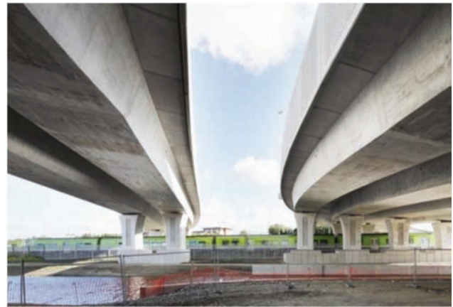
Figure 4.30 Example image of bridge with “prestressed concrete box beam multiple” superstructure. (Source: www.osdcconsultants.com.)
