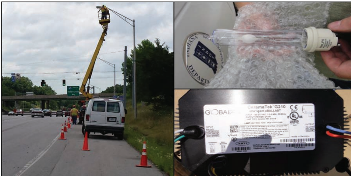
Figure 4.3 Field installation at Site 8, CMH lamp, and CMH ballast.
