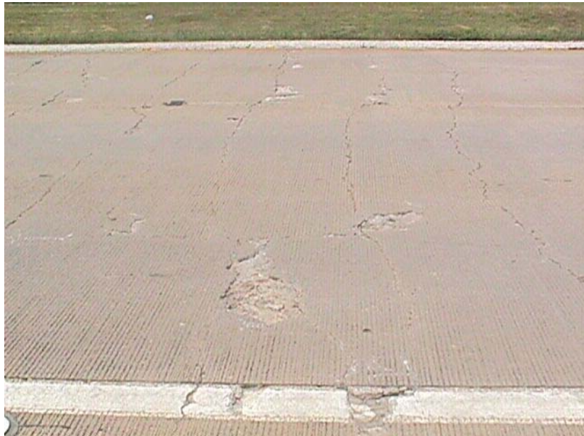
Figure 6.12 Typical severe spalls found in Section 13071-5
