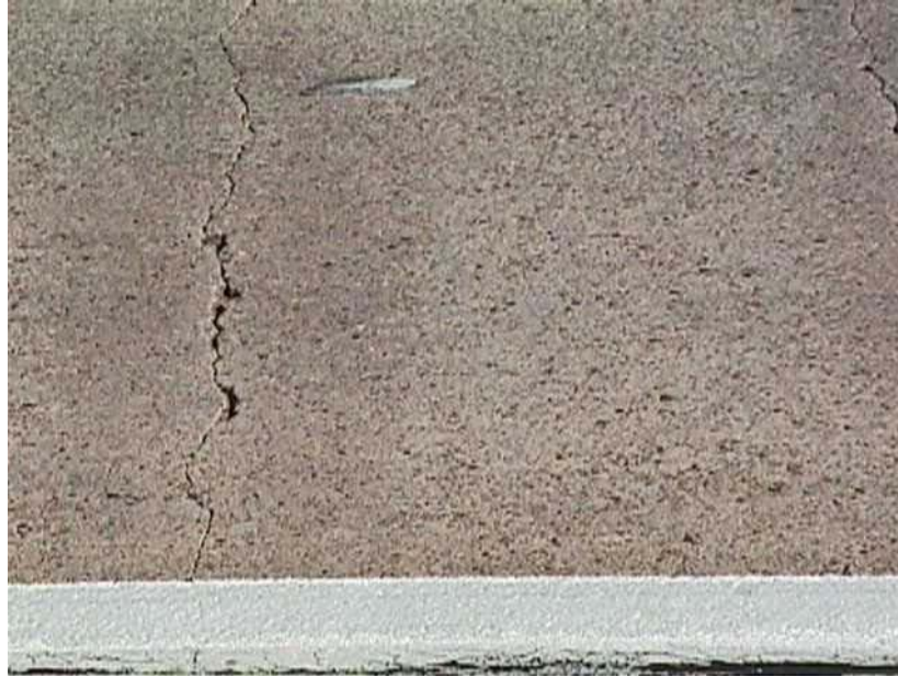
Figure 4.1 Isolated minor crack spall found in a CRCP
