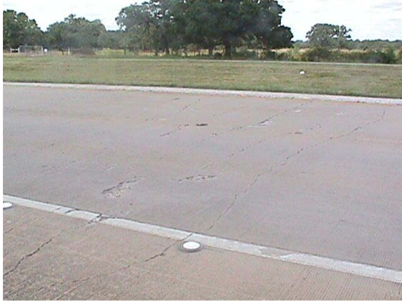
Figure 6.13 Another view of the spalls found in Section 13071-5
