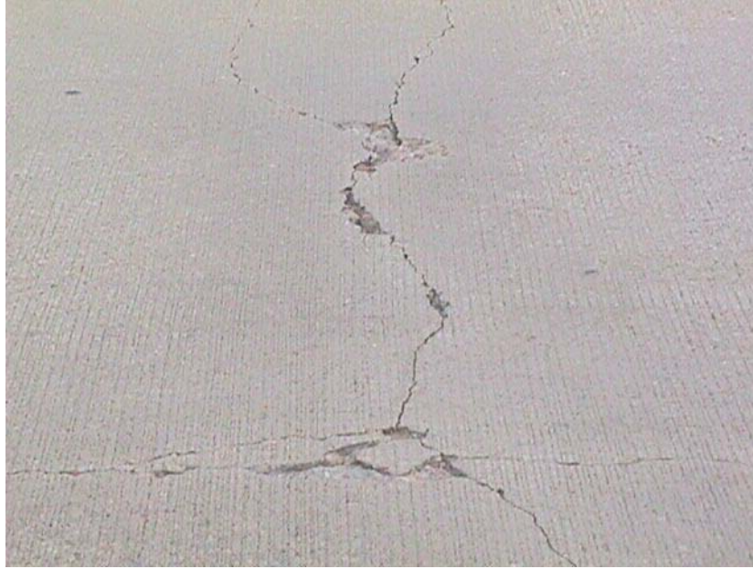
Figure 6.11 Severe spalls found in Section 13071-4
