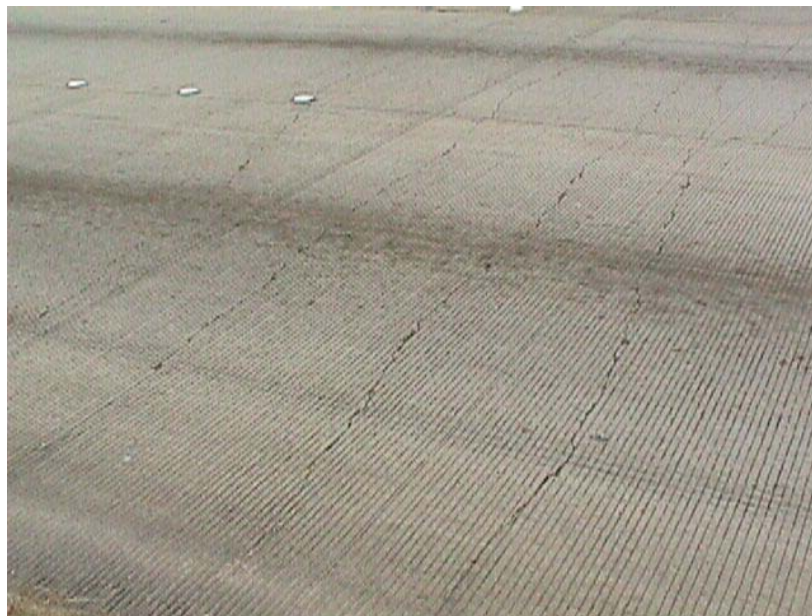
Figure 4.2 Series of minor spalls found in a CRCP on IH 10 in Houston
