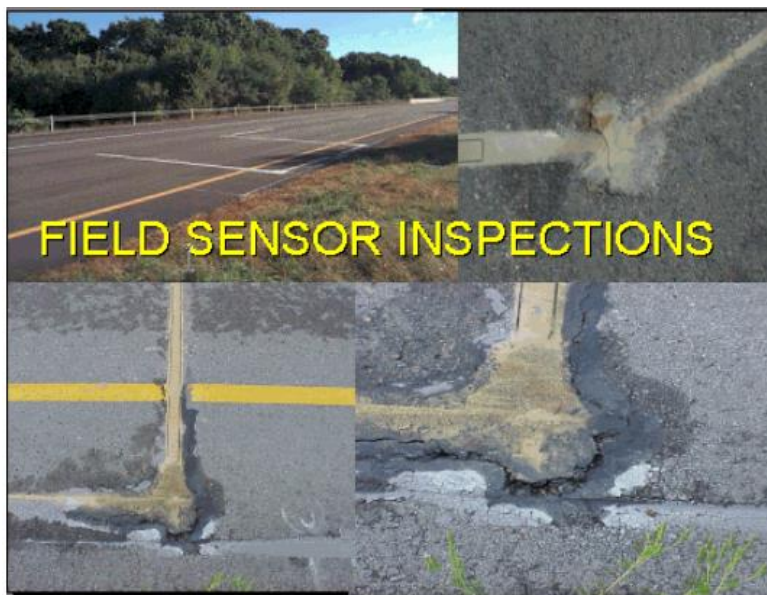
Figure 28: Field Inspection Images of Worse Case Conditions
