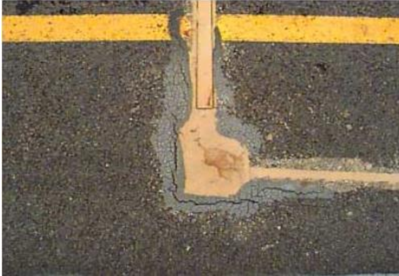
Figure 8A: Cracking Along End of Sensor Where Cables Exit Through the Conduits
