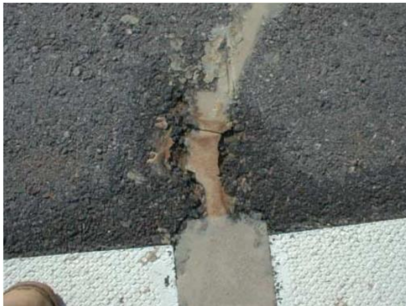
Figure 8B: Cracking and Pavement Deterioration At End of Sensor in Lane 2
