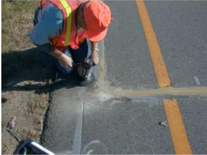
Figure 9: Grinding the Edge of Grout That Has Risen Above Shoulder Pavement Surface
