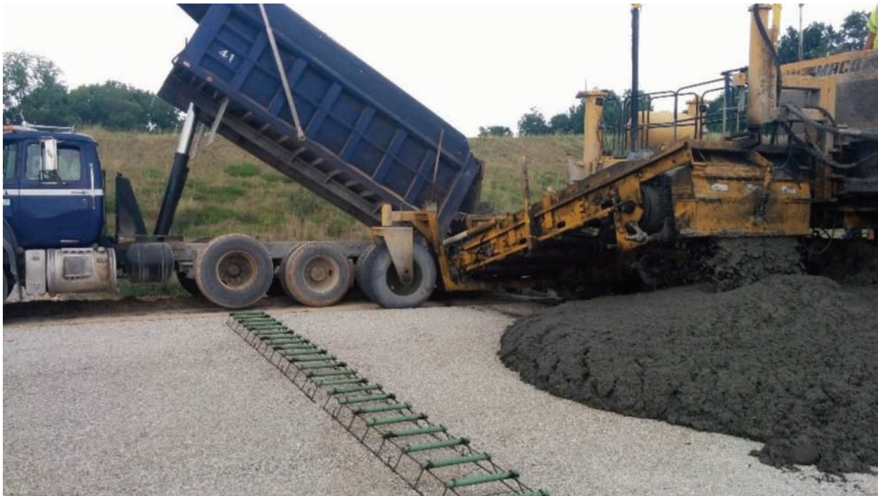
Figure 7.1 A photograph of the material in front of the paver, directly before sampling.
