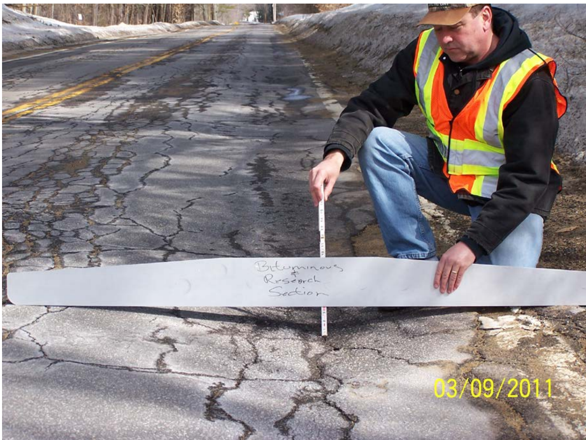
Existing Conditions – Deep ruts during frost heave season
