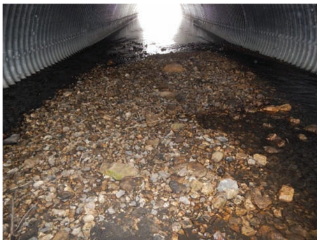
Figure 3.10 Image of STH80 CMP pipe-arch culvert over the Little Platte River, taken near the culvert inlet, and looking downstream.
