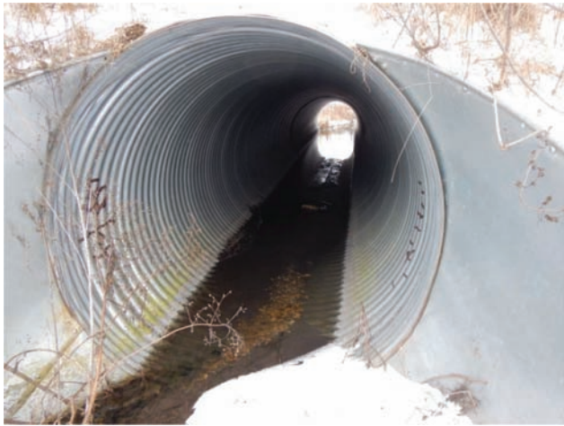
Figure 3.11 Image looking downstream of inlet of new embedded backfilled culvert installed about 300 ft to the east of the FHWA HEC-26 culvert.
