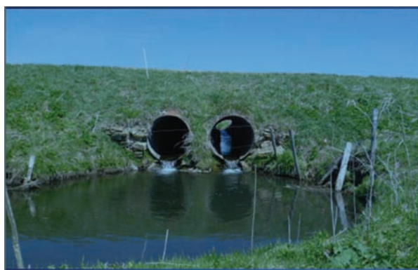
Figure 3.8 Perched outlet of pre-existing crossing structure with large scour pool. (Taken from Kirsch, 2014.)
