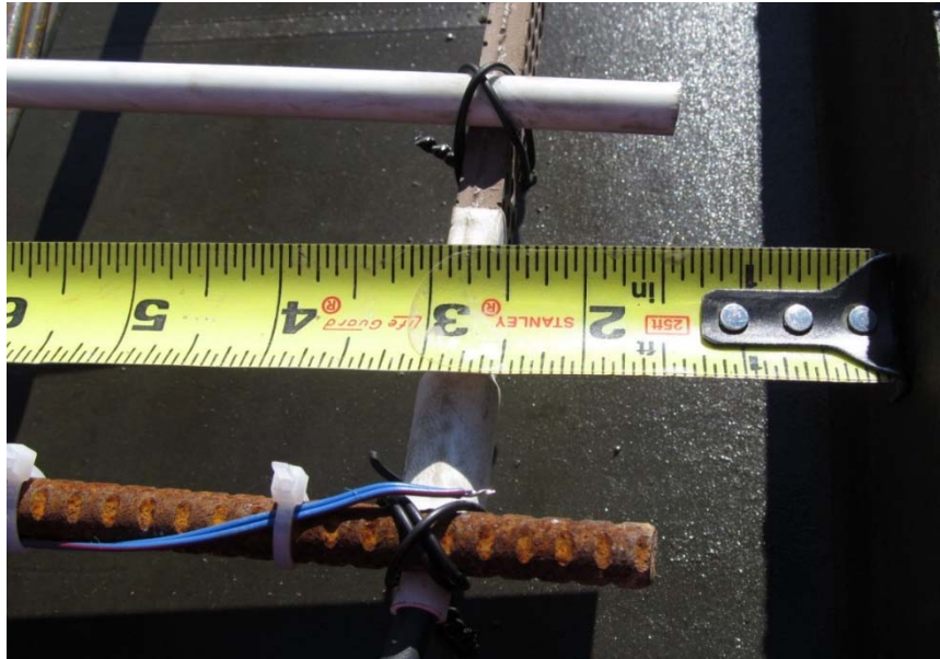
Figure 13 Thermocouple (blue wire) placed adjacent to embedded strain gage (Section B)
