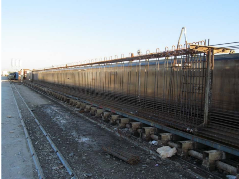
Figure 17 Stressed prestressing laid out for Girder 1 in the form beds at Gulf Coast Pre-Stress
