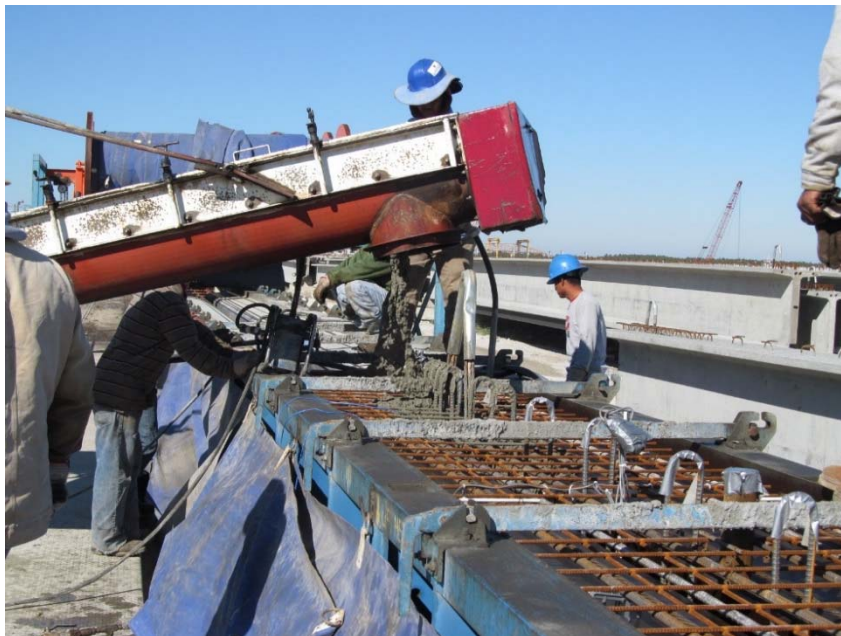
Figure 18 Concrete placement from the chute of a buggy into the forms for Girder 1
