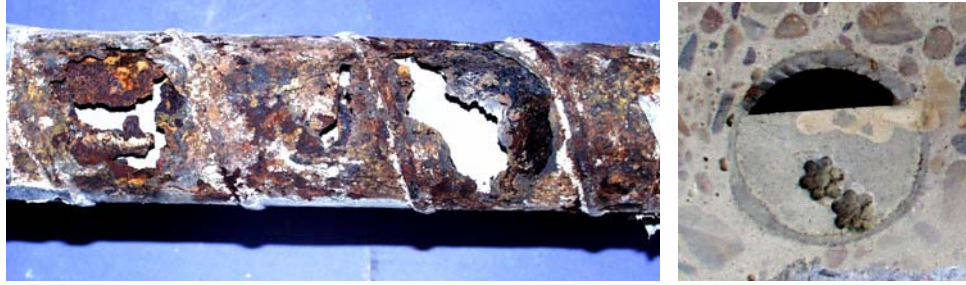
Figure 6.17 Bleed Water Void and Duct Corrosion 7
