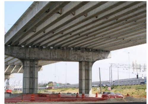
Excessive heat buildup can damage large concrete components if they are not correctly designed.
