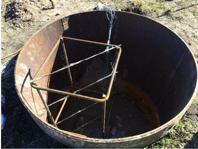
Figure E-4. Layout for frame for temperature logger attachment for shafts 2 to 4.
