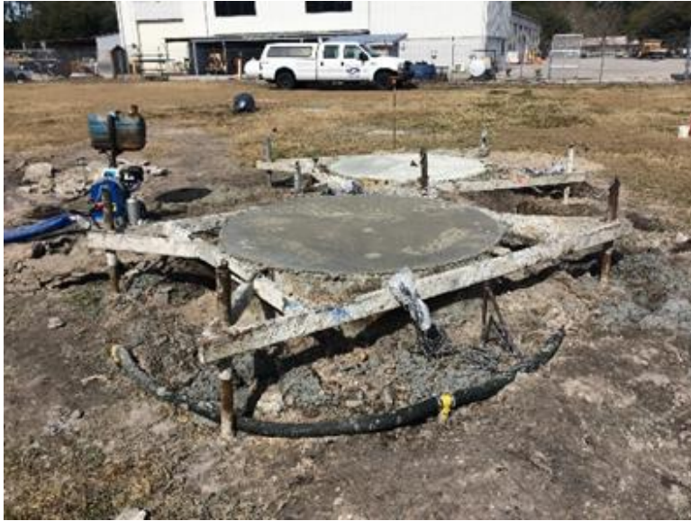
Figure E-11. Well field.
