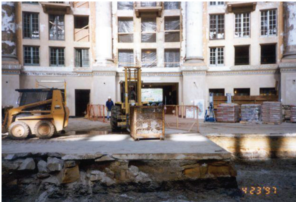
Figure A.2 Photograph of sulfate from shale causing disruption inside the West Baden Springs Hotel. (Courtesy of CFC, Inc.)
