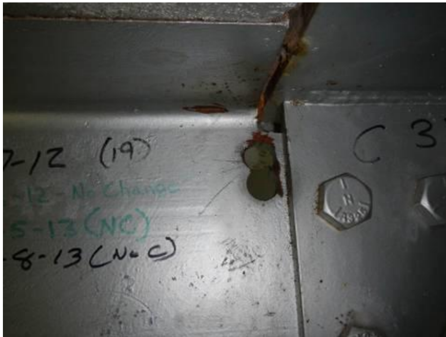
Figure 38. Multiple Holes Drilled at Fatigue Crack
