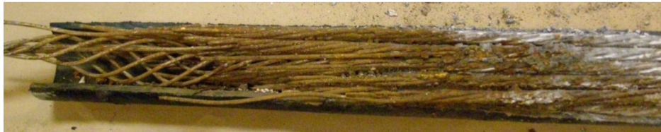
Figure 2.2. Strand corrosion at failure location. (Photo by author and courtesy of FDOT.)
