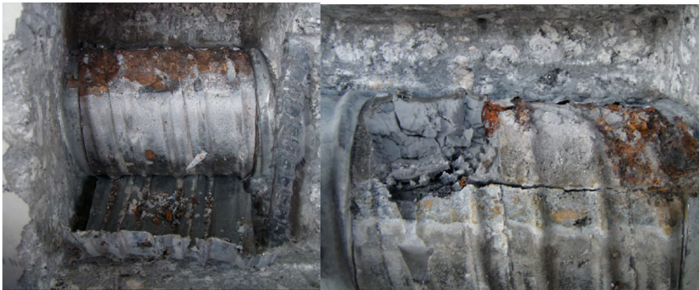
Figure 2.16. Corroded metal duct in vicinity of deficient grout. (Photos courtesy of FDOT.)
