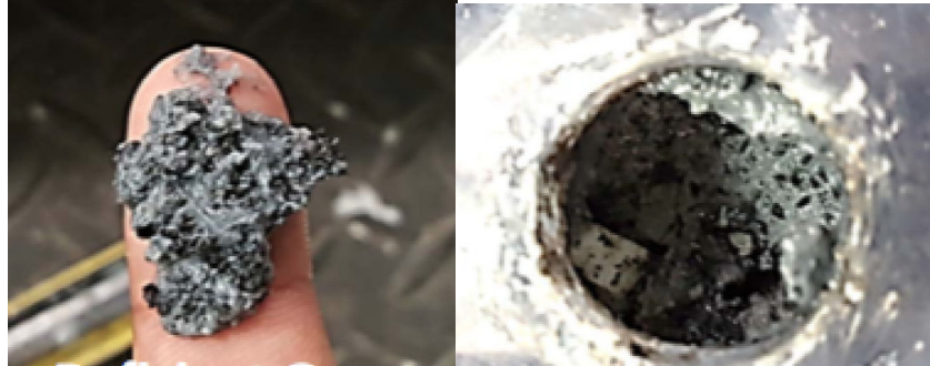
Figure 7.1. Photos of deficient grout from MIT test. (Location was adjacent to a probe location at ~0.3 ft. from the top of sample A)
