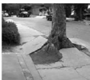
Less than 25% in Good Condition
