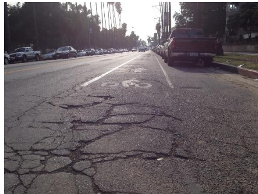
Bad Conditioned Bike Lanes 31
