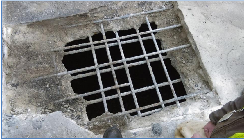
Figure 8: Bridge deck patch failure (Photo provided by Brandon Collett, ODOT District 8)
