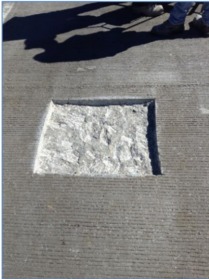
Figure 3: An example of a clean, smooth-cut hole, where patch #14 was installed (Lesak 2014)
