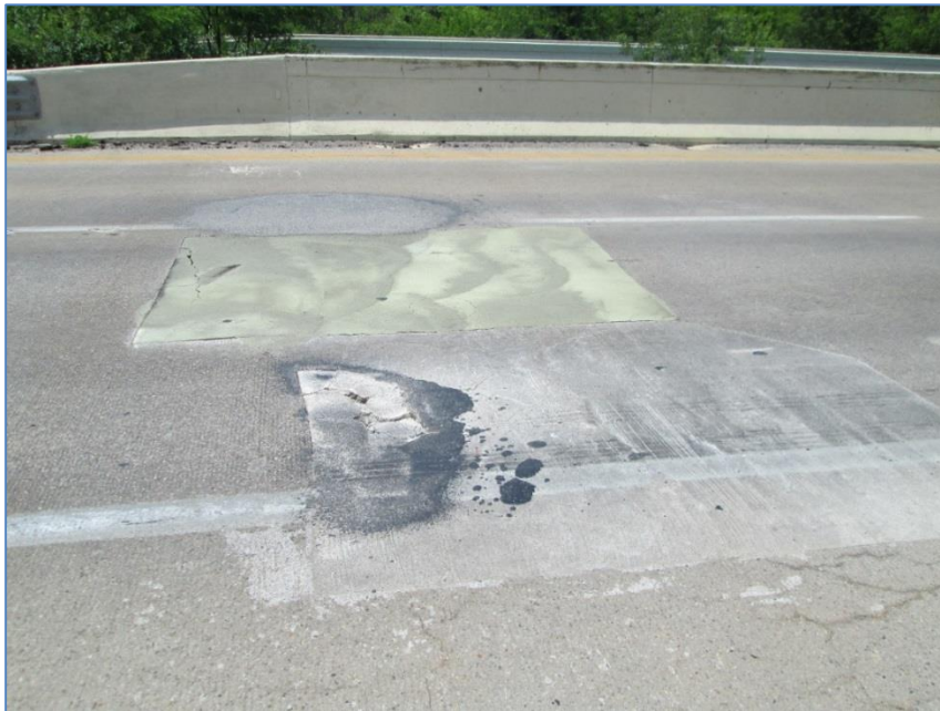
Figure 7: Condition of bridge deck patch in June 2015
