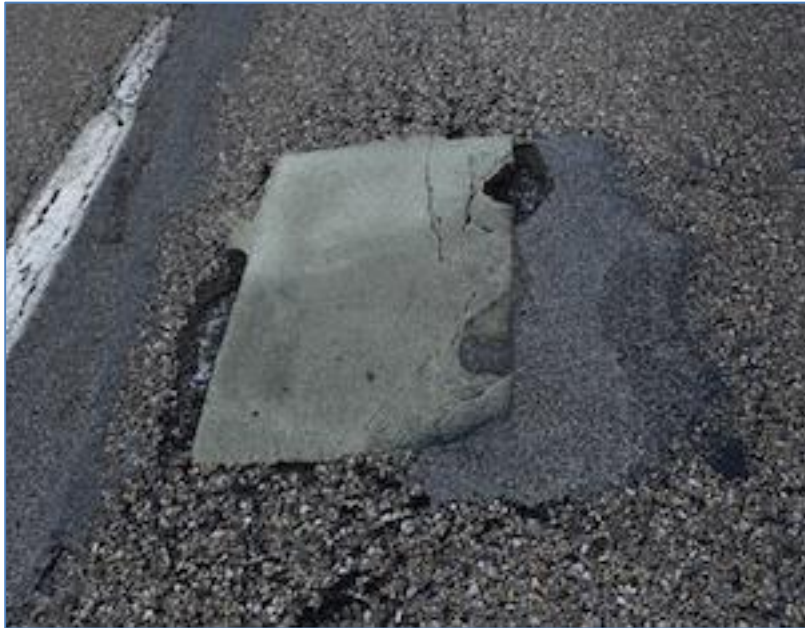
Figure 6: Example of failing patch in asphalt
