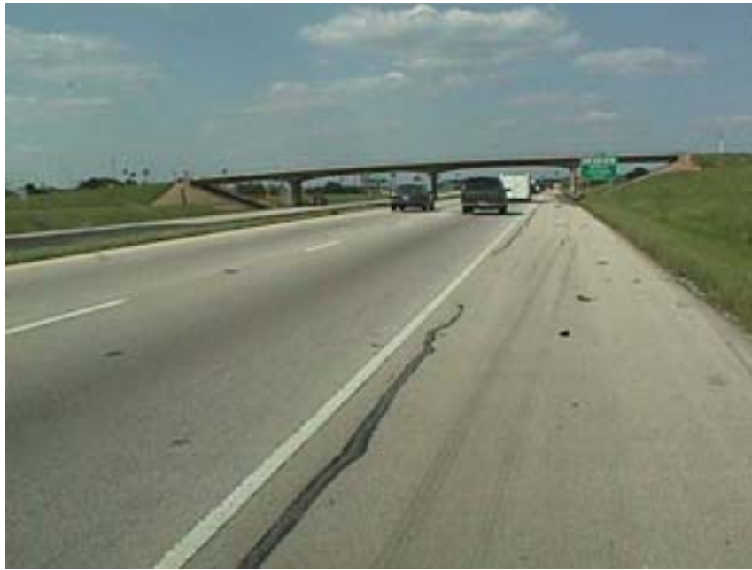
Figure 5.6 Longitudinal crack found between the outside lane and shoulder
