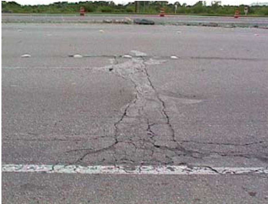
Figure 5.7 Failed patched area presenting alligator cracking
