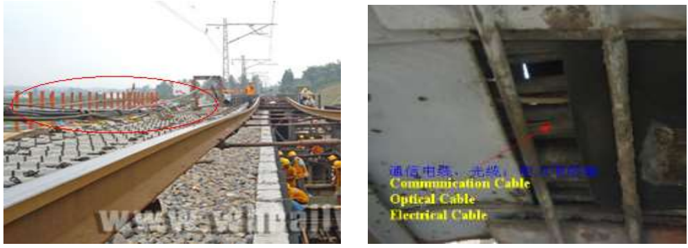
Figure 2.5.16 Movement of Cable Tray in Practice
