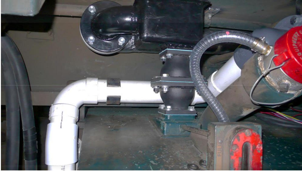
Figure 5. Exhaust pipe wrap-around the vent box
