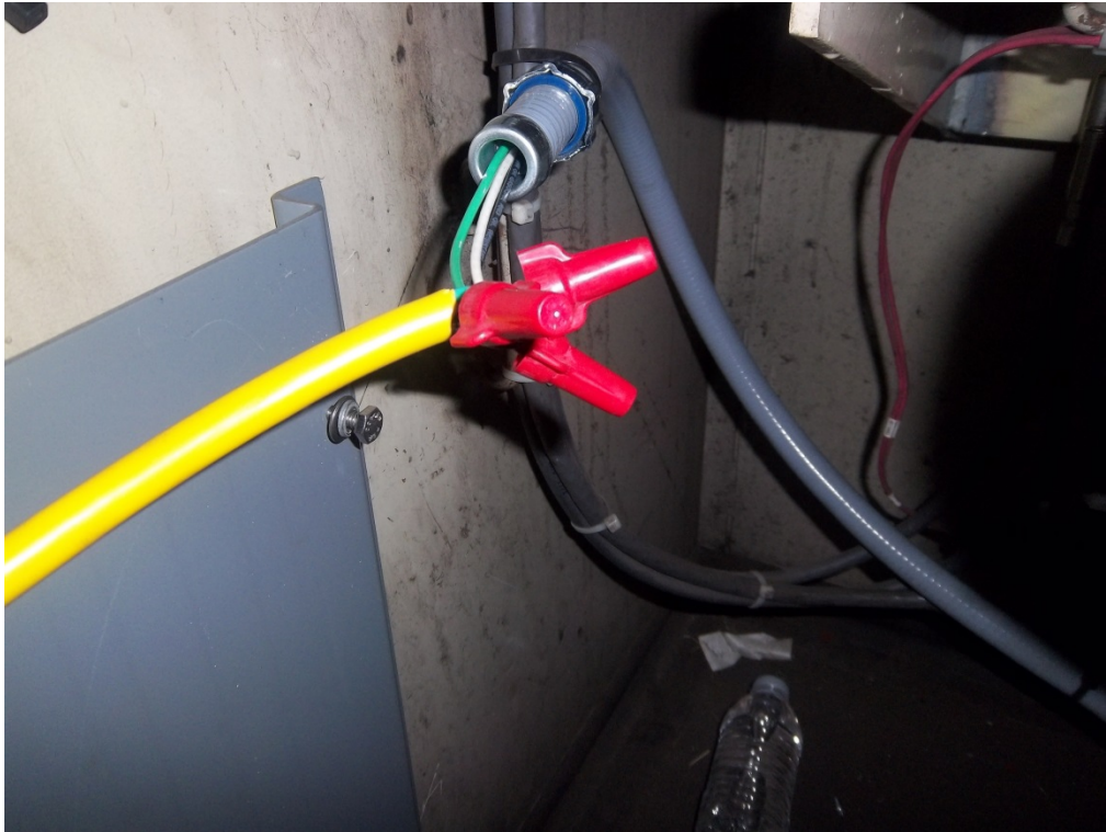
Figure 28. Power connection to the chiller from a separate source for functionality test
