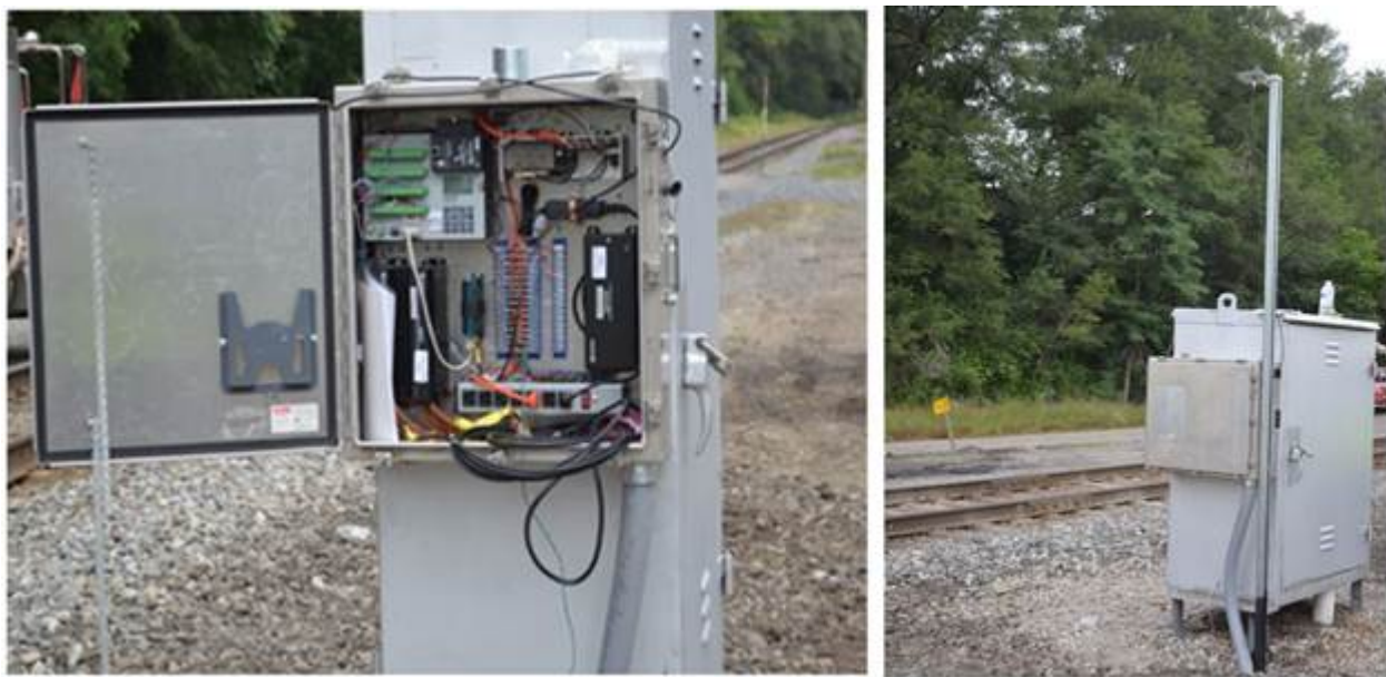
Figure 28. Instrumentation Logging and Remote Telemetry Box
