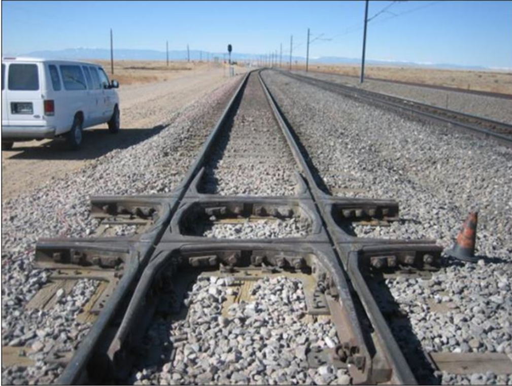
Figure 2. Cast Diamond Crossing Tested at FAST
