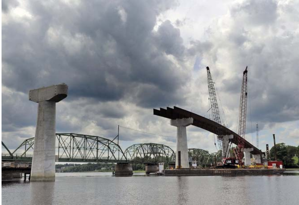
Figure 6.2: Image of the new bridge during construction in the foreground with the old bridge in the background (centralmaine.com, 2014)
