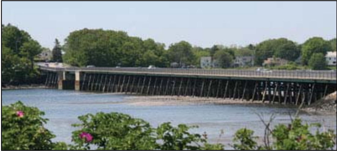
Figure 5.2: Martin's Point Bridge between Portland and Falmouth, Maine at the mouth of the Presumpscot River and Casco Bay during low tide (from MaineDOT 2013).
