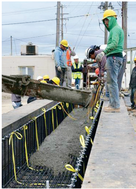
As part of an AASHTO Innovation Initiative, MDOT replaced the Plum Creek Bridge in Detroit with a CFRP-prestressed structure, a measure expected to reduce maintenance dramatically.
