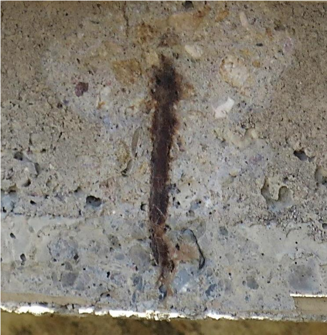
Figure 8.10 Spalling with exposed shear reinforcement on Girder C just south of midspan
