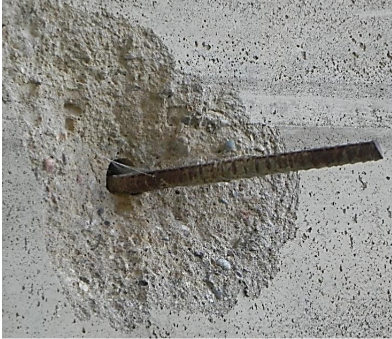
Figure 8.11 Large spalled region on Abutment 1
