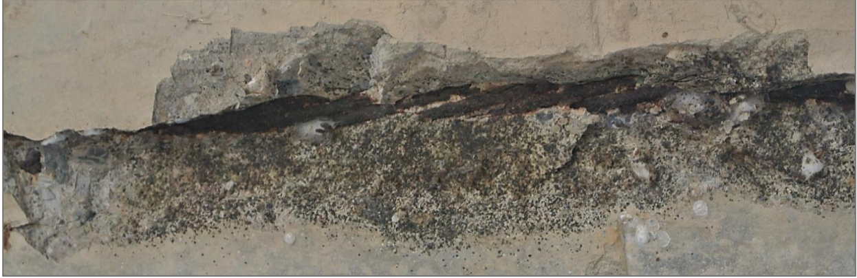
Figure 8.9 Spall on Girder C with exposed prestressing strand just south of midspan
