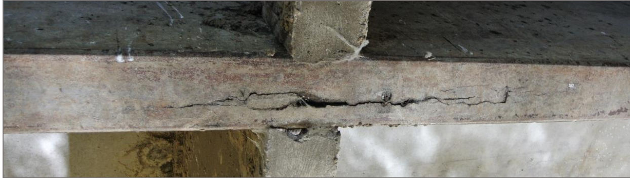
Figure 8.6 Longitudinal crack on Girder B at midspan
