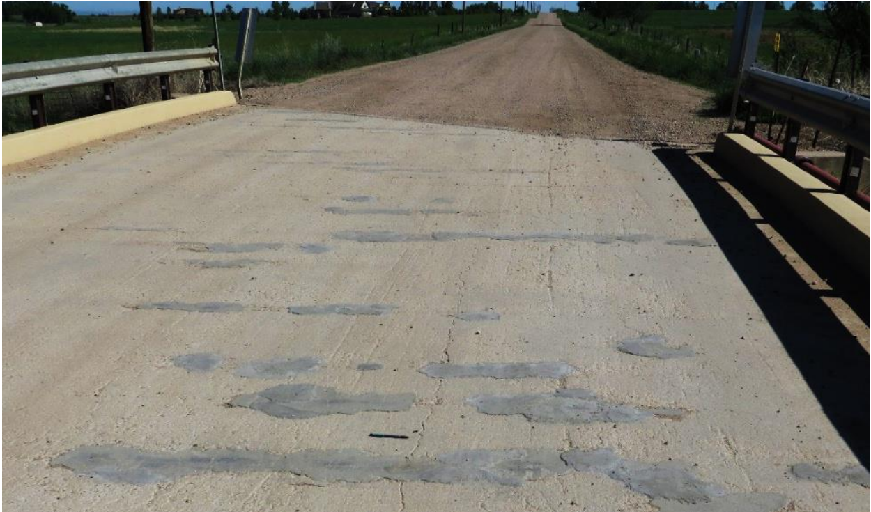
Figure 8.4 RC deck with longitudinal and transverse cracking
