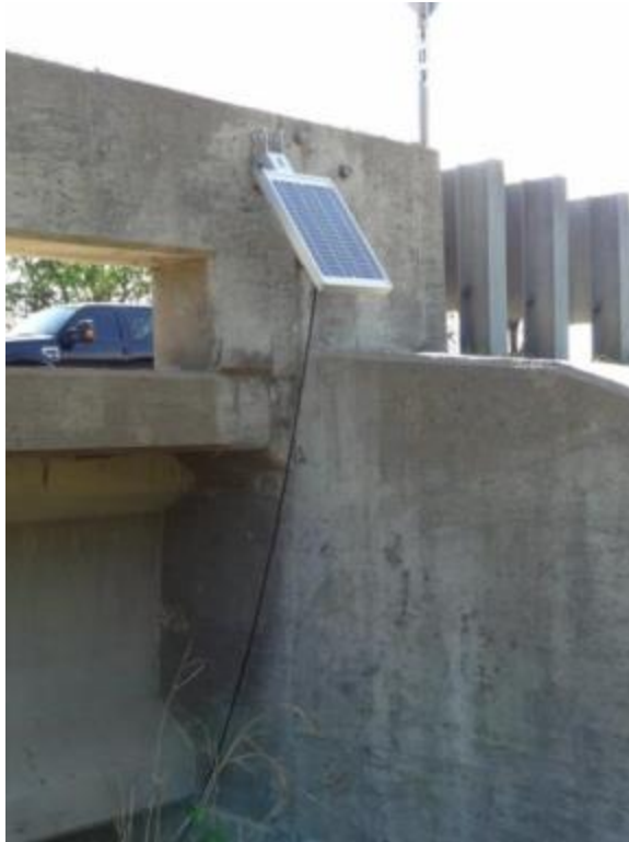
Figure 2.1: Solar Panel Mounted to Side of Bridge
