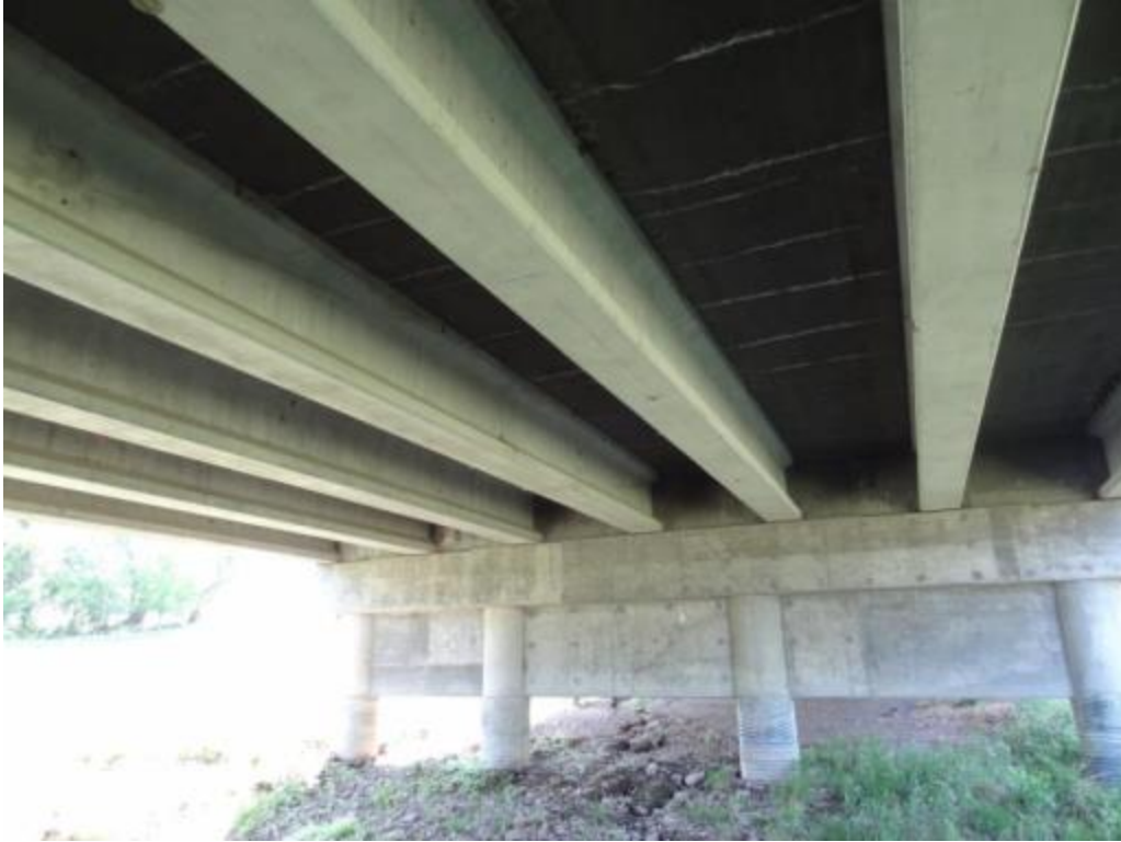
Figure 2.5: Typical View of Girders and Deck Showing Efflorescence
