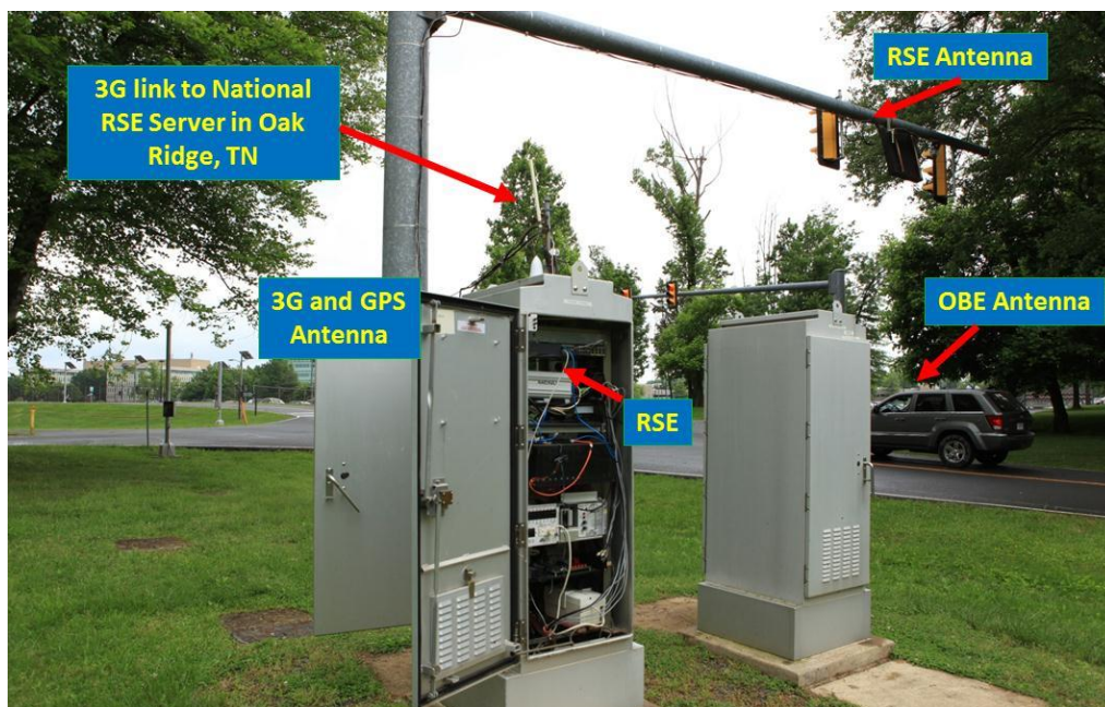
Figure 3-8. TFHRC's Cooperative Vehicle Highway Test Bed (CVHT) Intelligent Intersection (Source: Turner-Fairbank Highway Research Center, FHWA)
