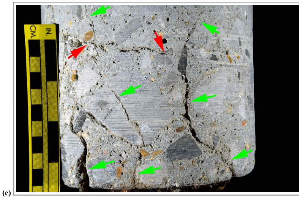
Figure A6 (cont'd). Photographs showing cracks on the side of the core. The red arrows indicate sub-horizontal cracks and the green arrows indicate sub-vertical cracks.
