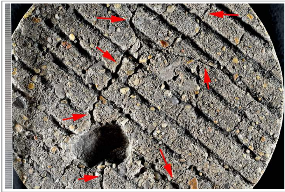
Figure C5. Photograph of the top surface showing overview of cracks (red arrows). Scale in millimeters.
