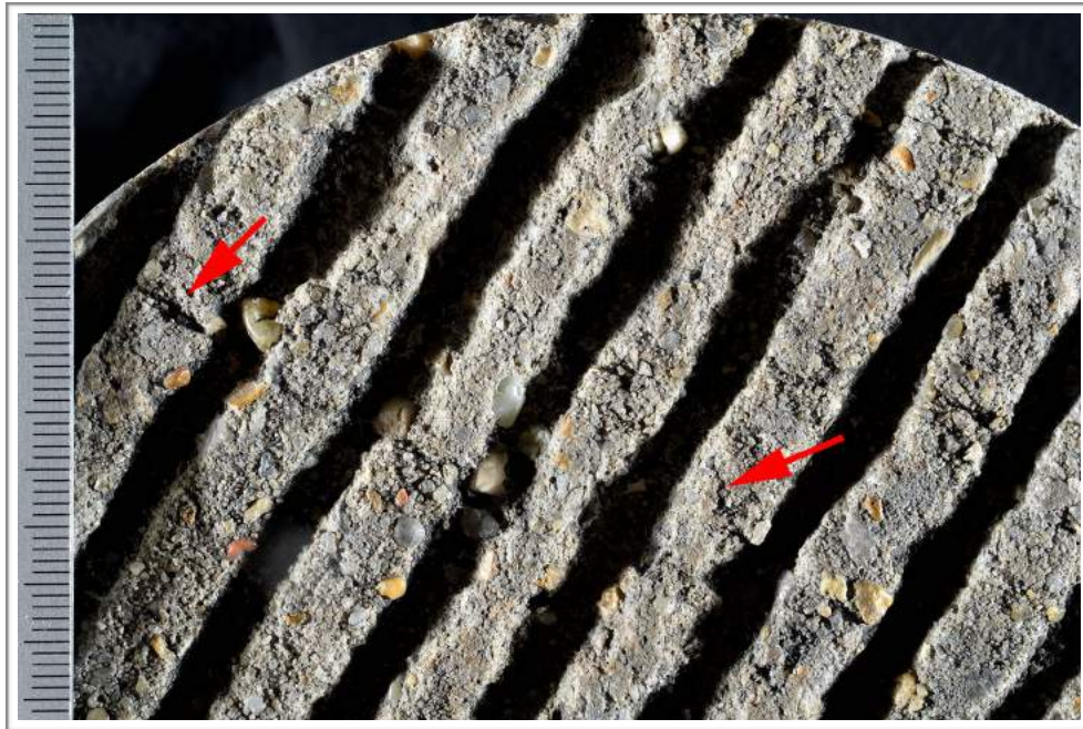
Figure A5. Photograph of the top surface showing linear cracks (red arrows). Scale in millimeters.
