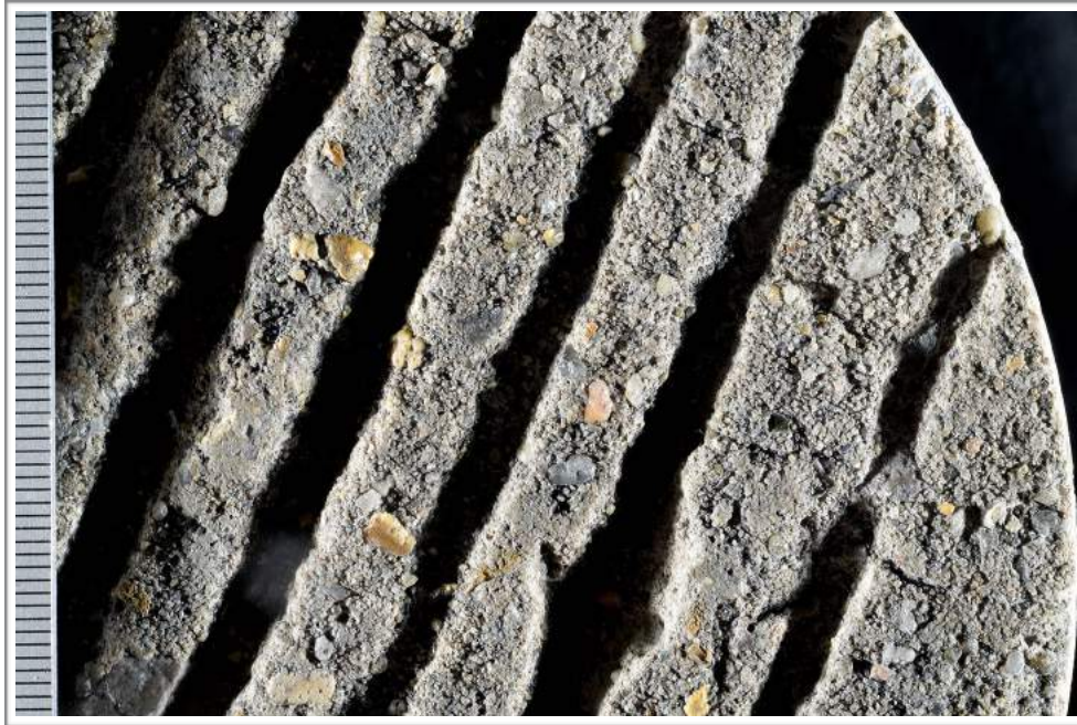
Figure A3. Photograph showing detail of tined top surface; scale in millimeters.
