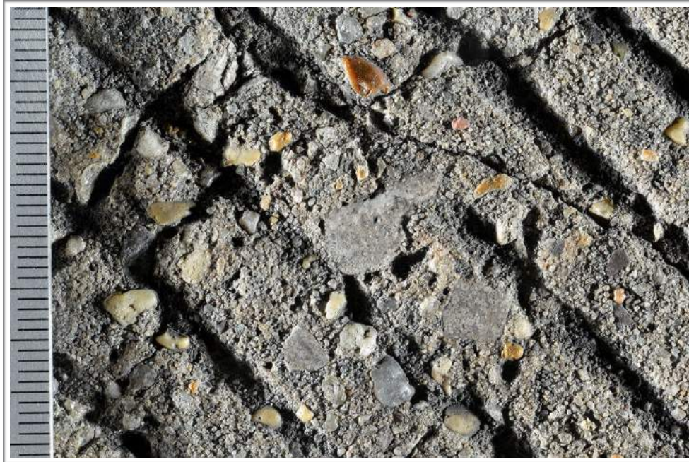
Figure C3. Photograph showing detail of top surface; scale in millimeters.
