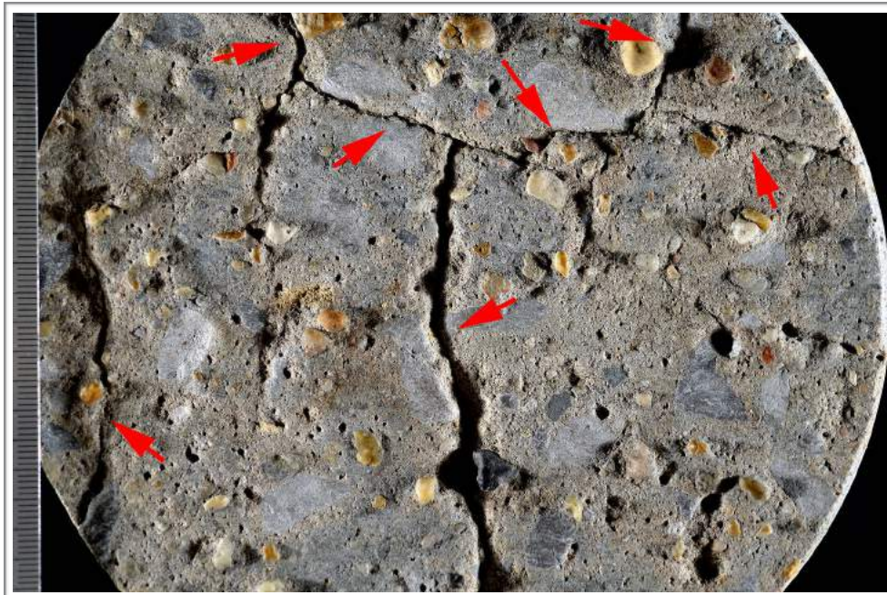
Figure B4. Photograph of top of core showing cracks (red arrows); scale in millimeters.
