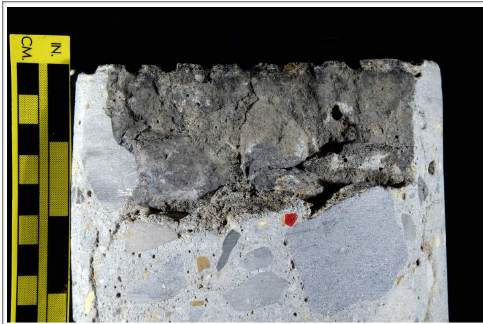
Figure A4. Photograph of top of core showing missing section.
