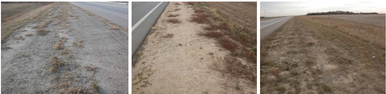
Figure 1-1. Problematic sites on Nebraska Highway 34, 41, and 275 (left to right).
