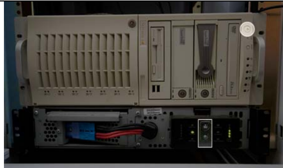
Inside right door of main electronics cabinet
