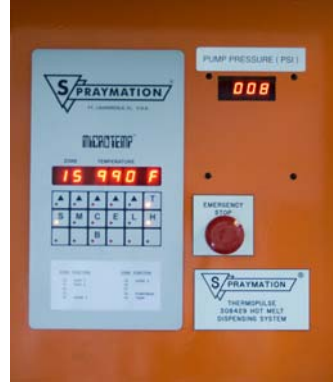
Inside hot-melt adhesive system cabinet
