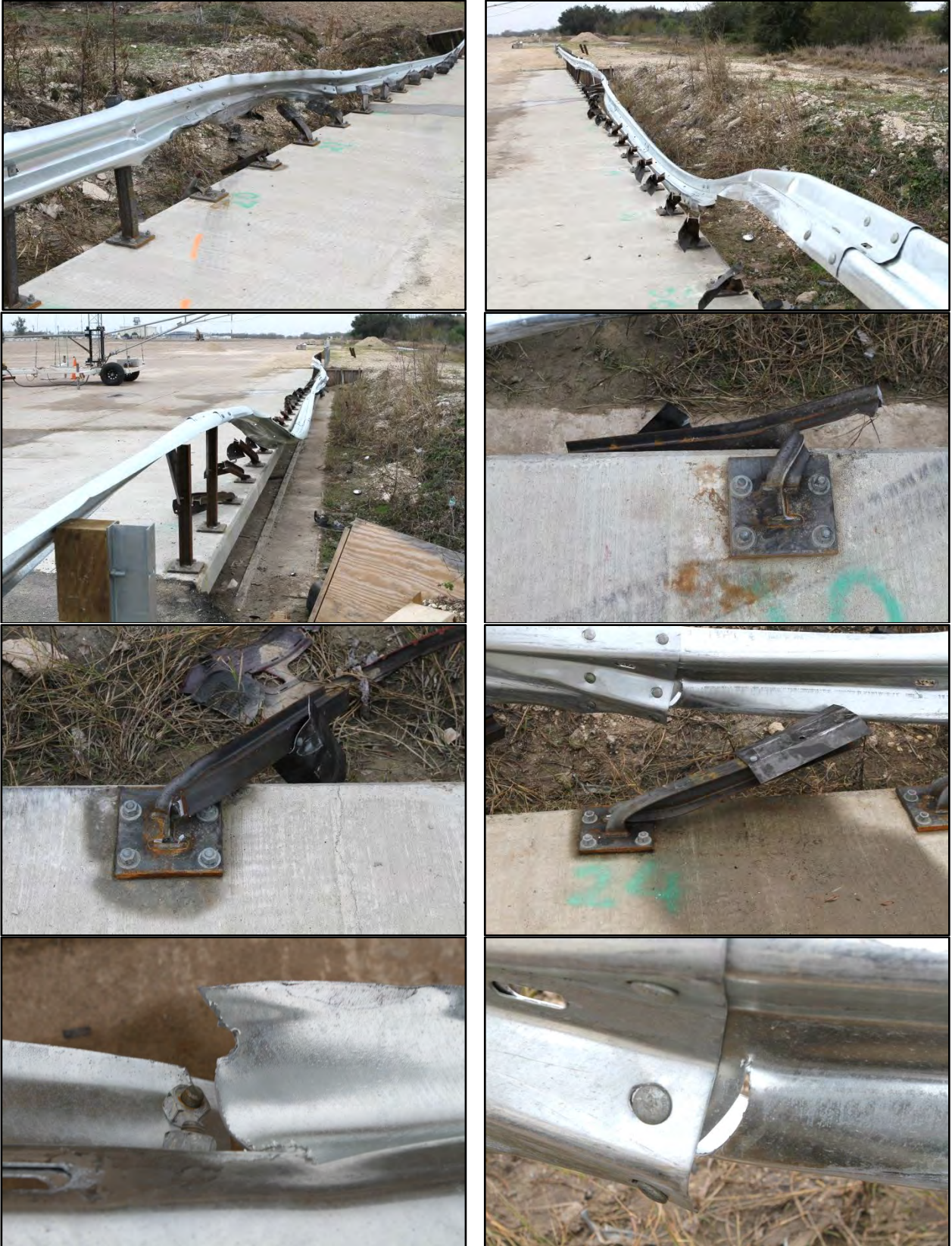
Figure 5.4. TxDOT T631 Bridge Rail after Test No. 490024-1-2.
