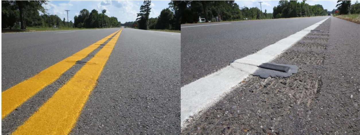
Figure 12. CLRS with Rumble Bars (Left), ELRS with Rumble Bars (Right).
