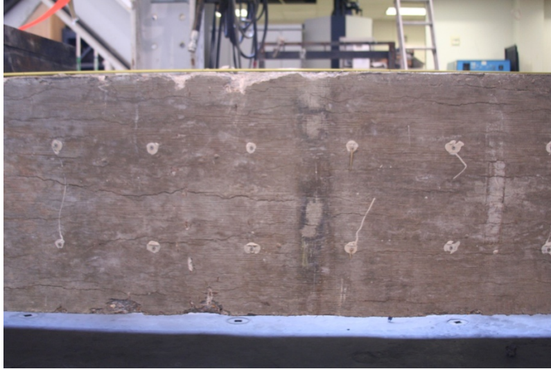
Figure 3-7. Cracking of Specimen #1 prior to Structural Load Testing.
