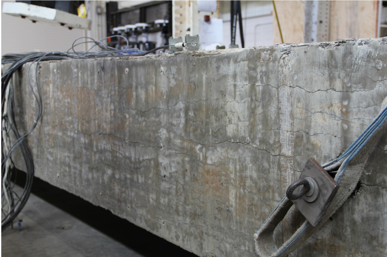
Figure 3-9. Cracking of Specimen #12 prior to Structural Load Testing.
