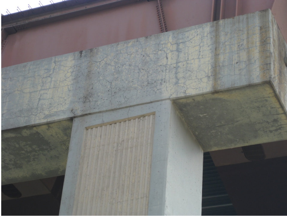
Figure 2-3. Cracking in Bent Cap under Minimal External Loading (Houston, TX).
