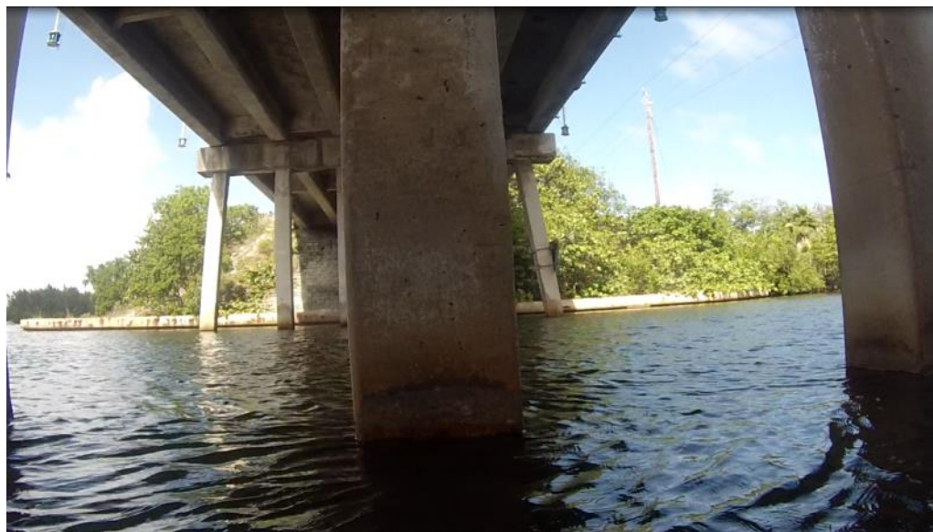
Figure 43: Example splash zone images of bridge structures acquired using the hull-mounted digital video camera.
