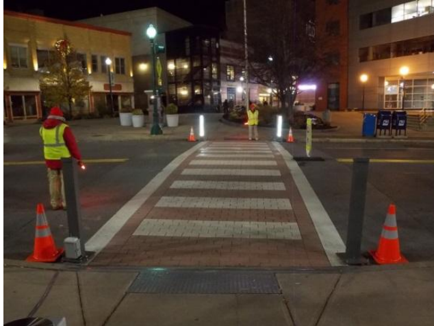
Figure 10. Illuminated appearance of bollard crosswalk lighting system at night.
