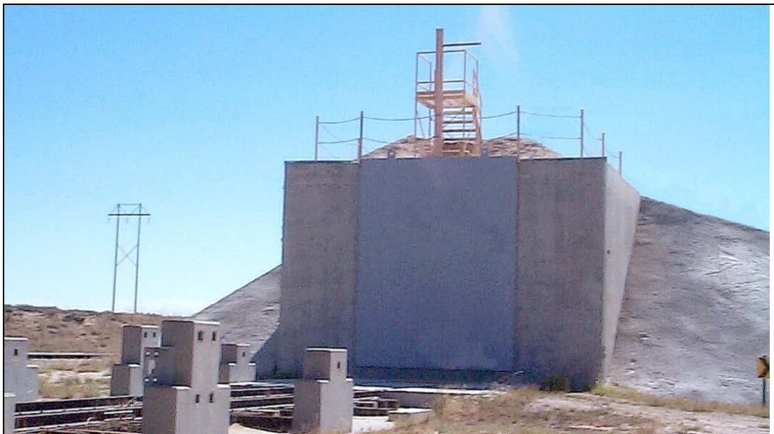
Figure 45. Vehicle Impact Wall
