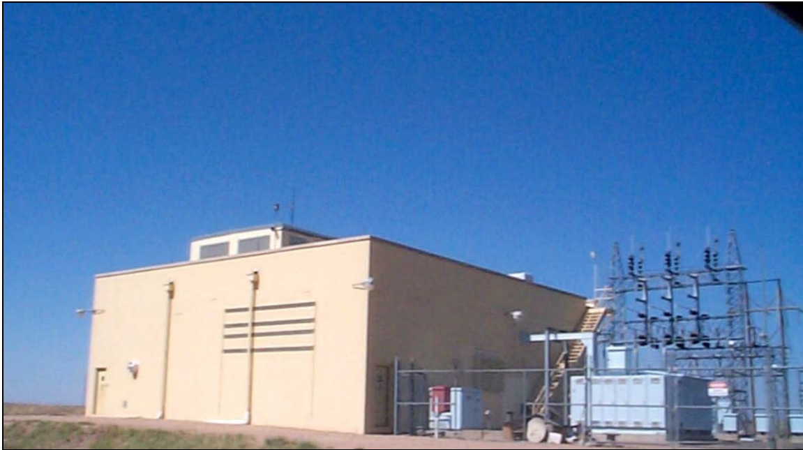
Figure 19. DC Rectifier Substation #1
