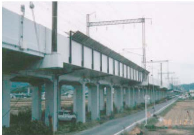
Figure 13. Barrier to mitigate noise and pressure pulse affecting buildings close to the track, from Kikuchi et al [48]
