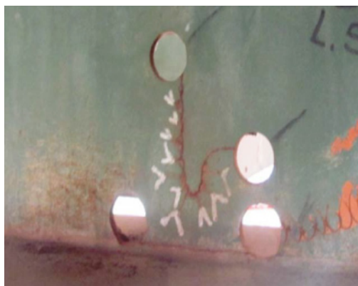
Example of the Types of Cracks Occurring in Kansas Bridges
